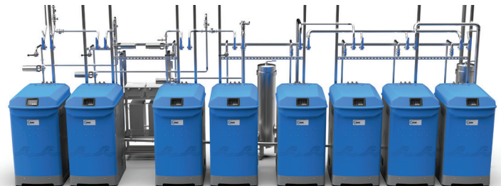
WFI Generation System
